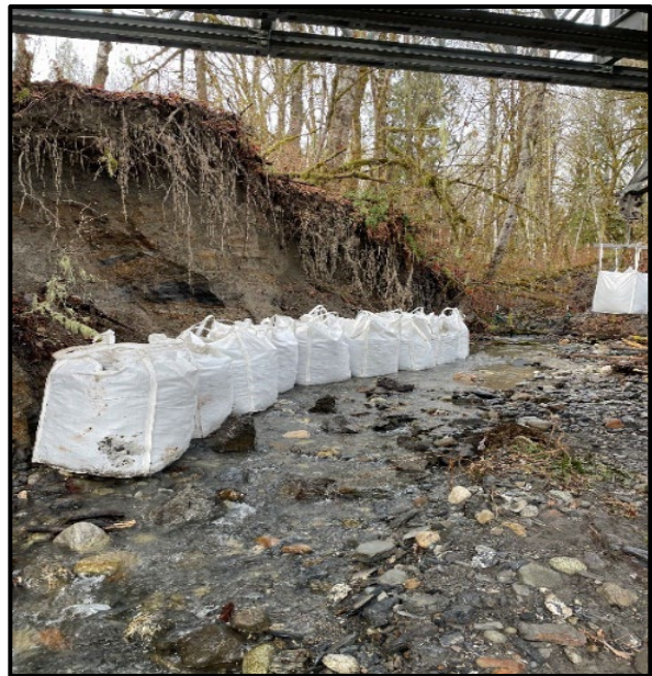
Super-sacks filled with stream gravel are placed to armor bank and slow down channel migration.
