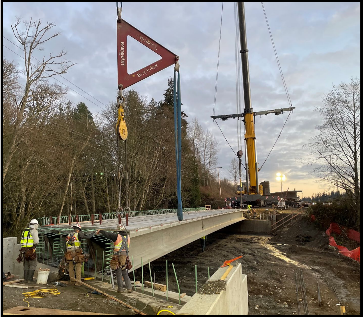
Construction of the new “Cedardale Road at Fisher Creek” crossing, installation of the 133-foot long pre-stressed concrete girders, December, 2024.
