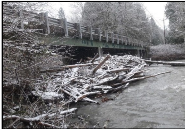
South Skagit Highway at Finney Creek
