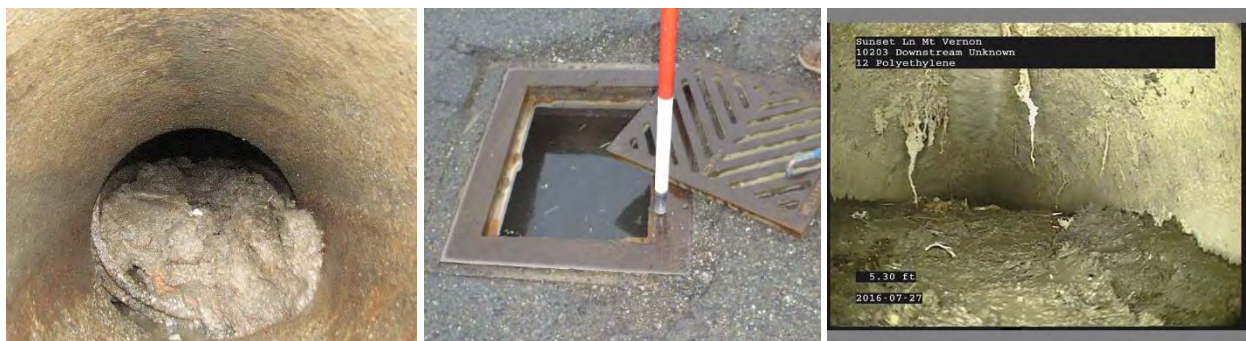
Figure 7: Sediment Plugged Pipes in Dunbar Road and Highway 536 Intersection (left and middle, January 26, 2016; right, July 27, 2016)
