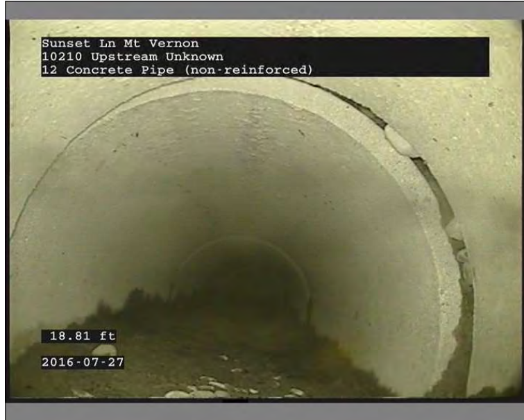
Photo: Unknown1021027072016_125738.JPG 18.67FT, Joint Separated Medium
