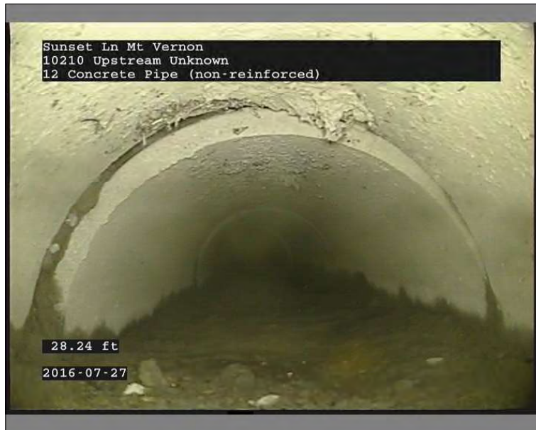
Photo: Unknown1021027072016_125838.JPG 28.24FT, Joint Separated Medium
