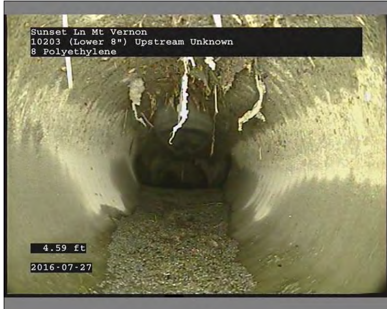
Photo: Unknown10203 (Lower 8)27072016_114017.JPG 4.11FT, Deposits Settled Fine, 15 %of cross sectional area, from 04 to 08 o'clock, , within 8 inches of joint: YES, Start
