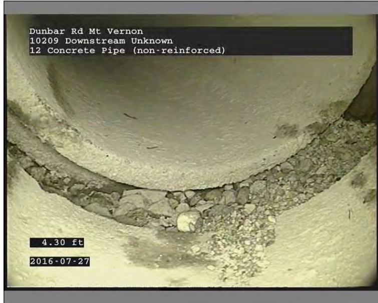
Photo: 10209Unknown27072016_143844.JPG 4.3FT, Joint Separated Medium
