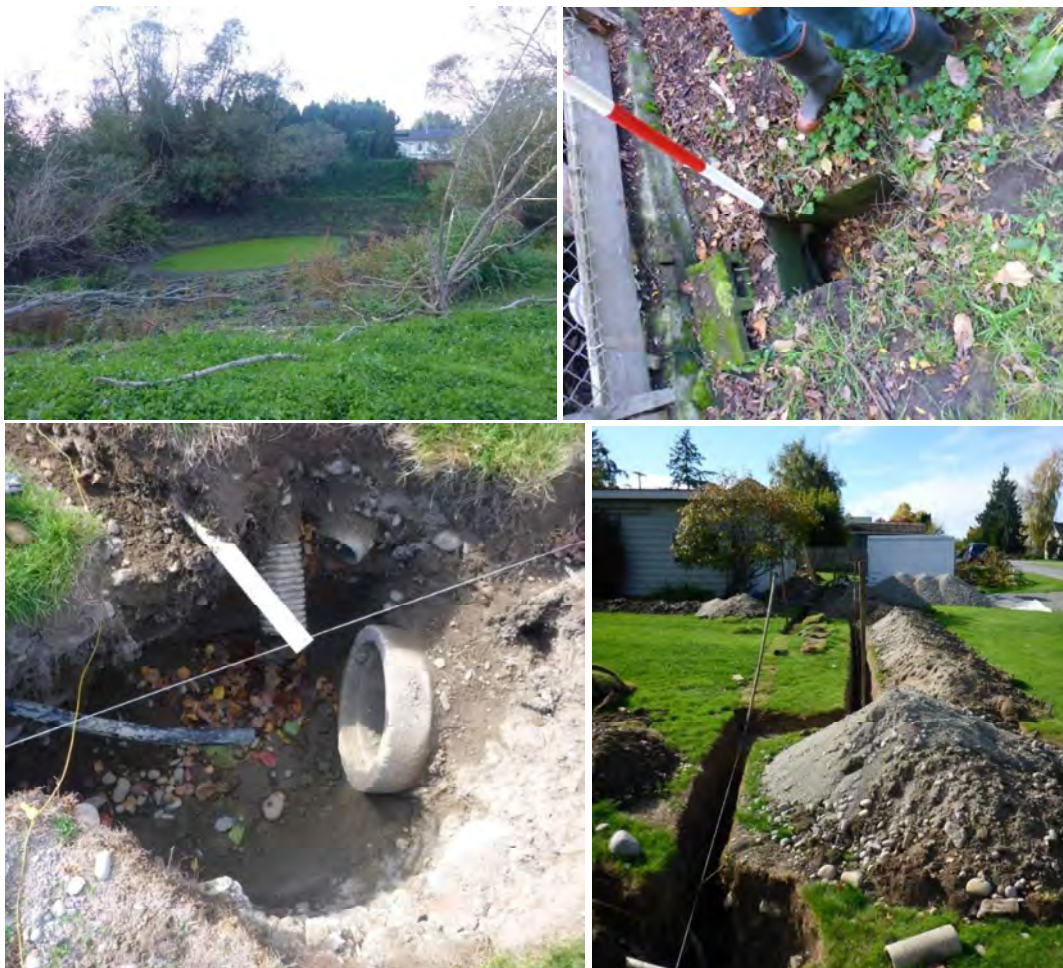
Figure 5: Pond on East Side of Sunset Lane (upper left, pond; upper right, pond inlet; bottom left upstream end of inlet pipe; bottom right, exposed yard drains connected to pond inlet)
