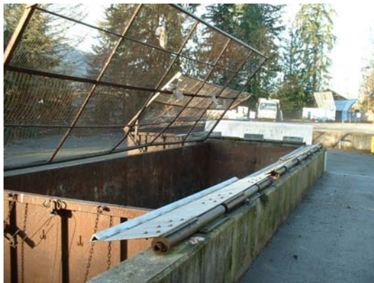
Figure 4 Sauk Waste Drop Box
