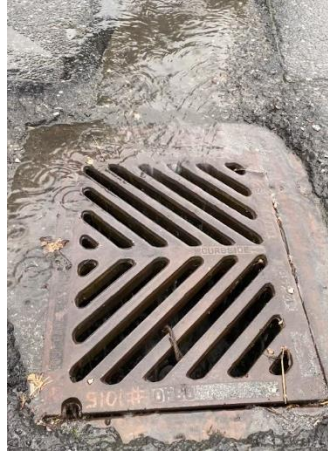
Figure 1-1. Stormwater runoff flowing into a storm drain before making its way to the Skagit River.
